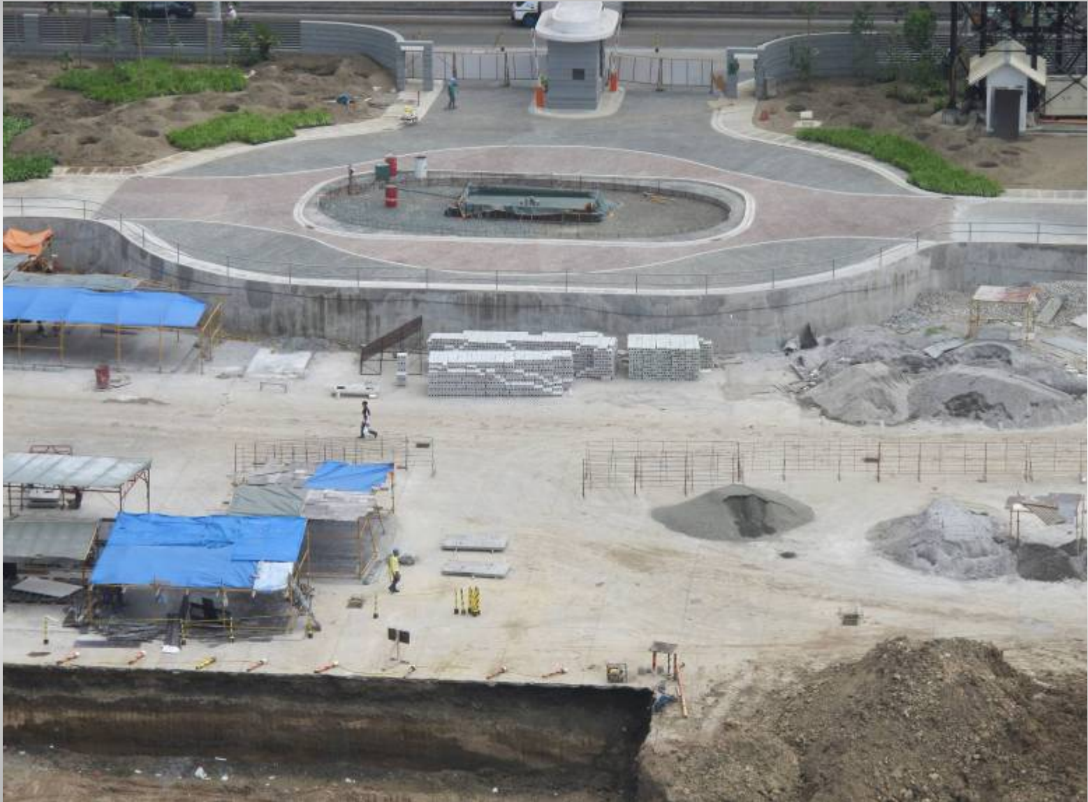
A view of the arrival area, completed guard house and on-going construction of the water fountain and man-made beach
