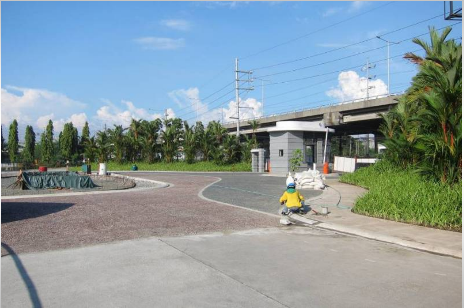
A closer view of the paved arrival area with the beginnings of the water fountain on the left and guard house on the right
