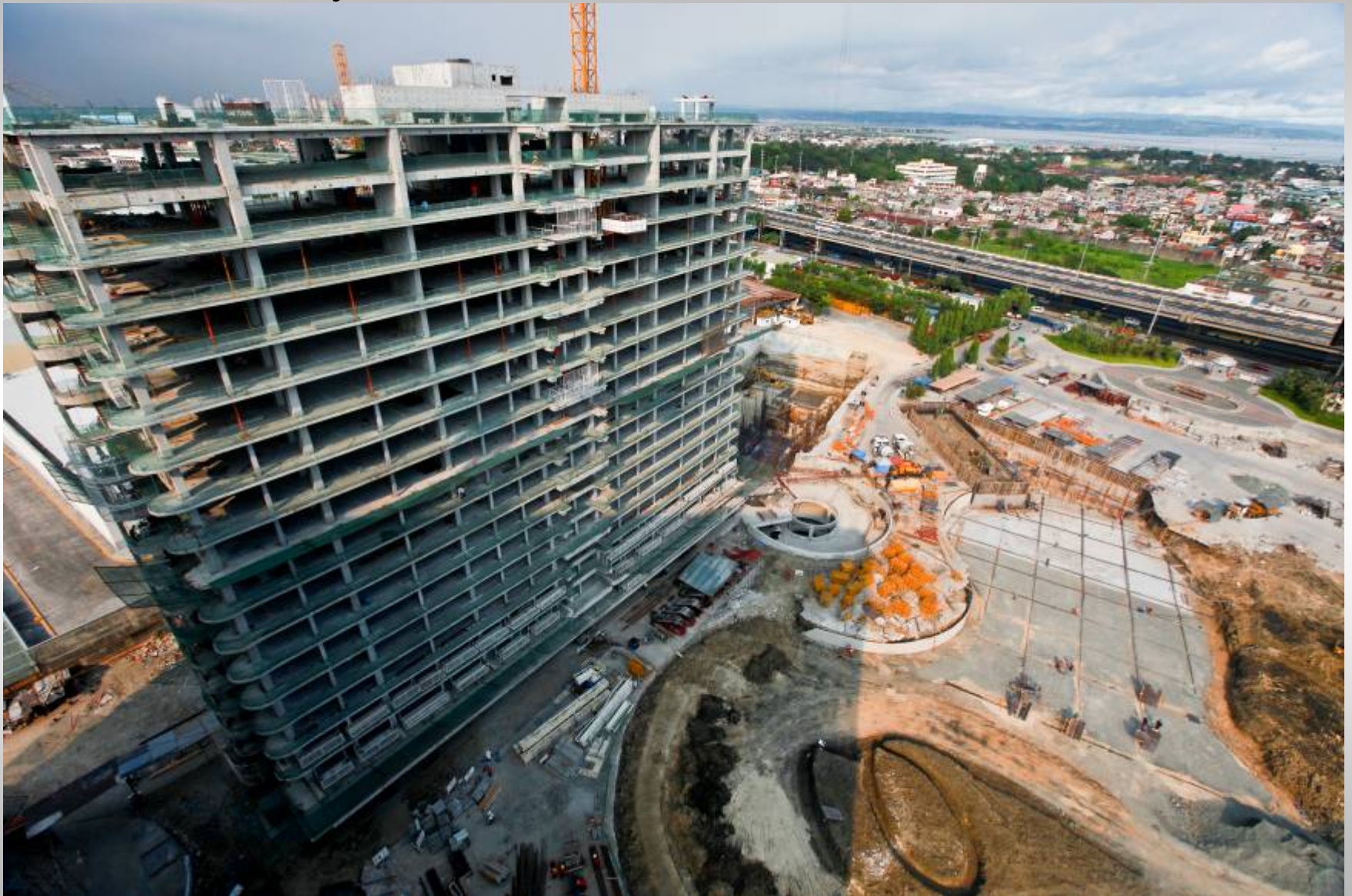
A closer look at Santorini tower with the circular ramp on the right leading to basement parking levels
