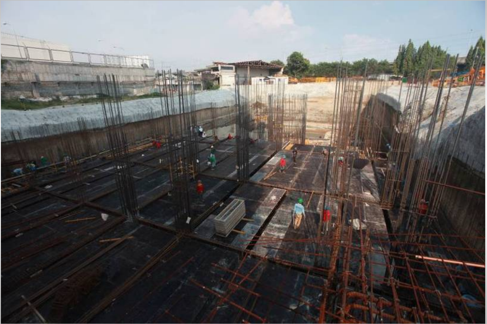
Formworks and rebar installations are in progress at the basement parking levels of St. Tropez, the third building rising at the Azure.
