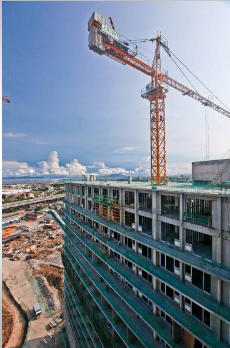
The Rio's roof deck and the ongoing balcony installations in the upper floors
